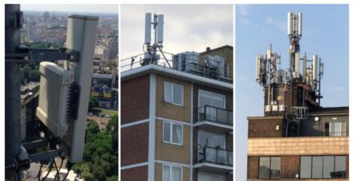
Figure 17: Small cell (Rooftop tower)
