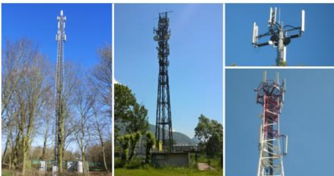
Figure 16: Macro BTS (Ground-based tower)
